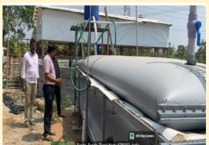
Field visit to Bio-Digester unit (KVK, Erode, TN)
