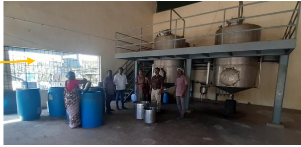
Oil Distillation Unit
