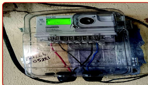
IFS-Solar On Grid Running Status
