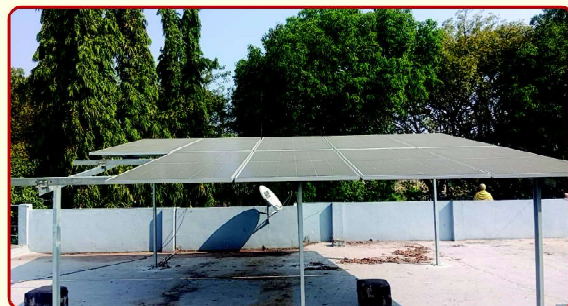
5KW Solar on-grid power system
