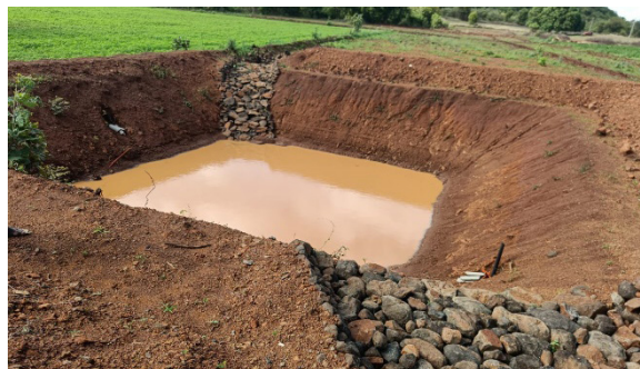
Demonstration of water harvesting structure ICAR-CRIDA, Hyderabad
